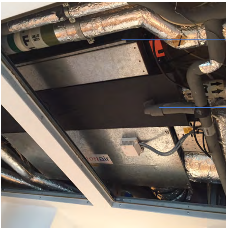
Photo 9: locating the condensate drain and filter
